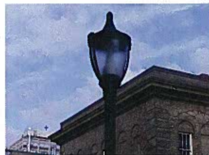
Former HID fixture after its LED retrofit
