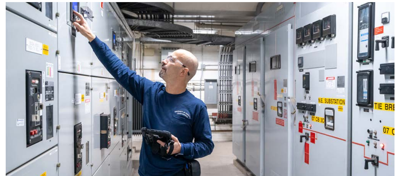
F&S teammate Peter in electrical substation (photo by Donglin Que)
